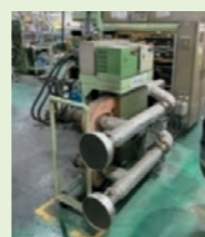
Electric hot-air generator
