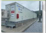
Tagawa Energy Storage Plant (Kawara Town, Tagawa-gun, Fukuoka Prefecture)
