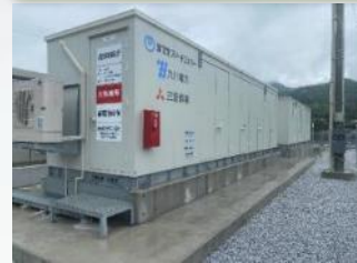
Tagawa Energy Storage Plant (Kawara Town, Tagawa-gun, Fukuoka Prefecture)
