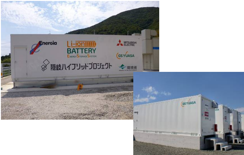
Power storage system
