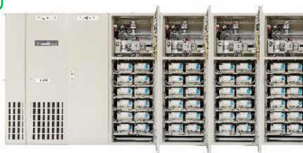
[Storage battery systems]
