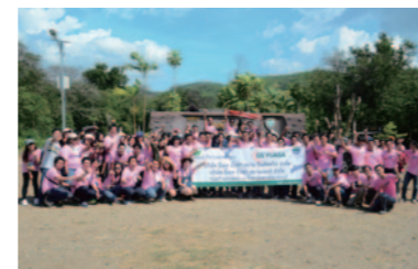
Participating in the construction of a dam (as a measure against flash floods during the monsoon season)
