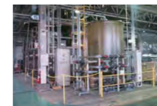
Water recycling equipment
