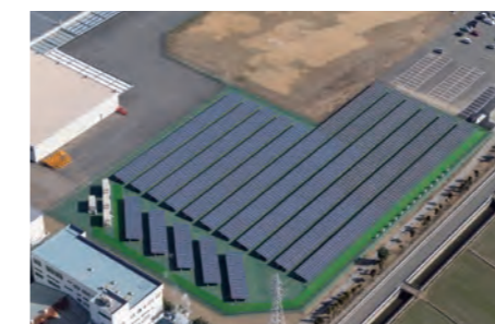
Full view of the mega solar installation
