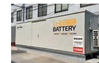
Exterior of an ESS container
